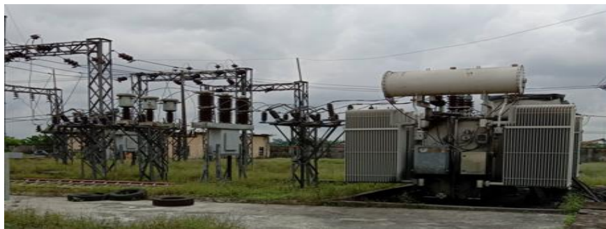
Figure 9. Otovwodo 15 MVA injection transformer and switch yard
